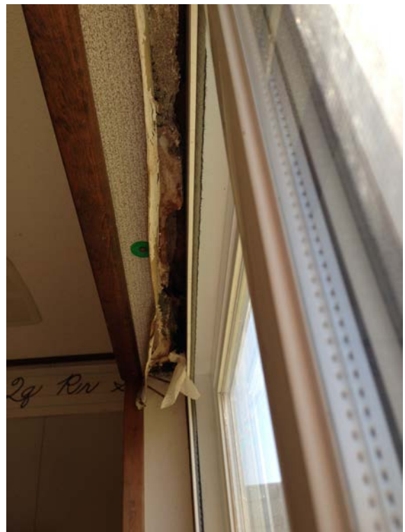
Window loose from Rotted Wall
